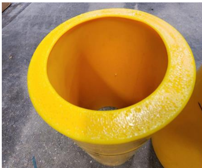
Figure 4. Example of small bubbles observed in the fusion zone of PA12 pipe. While such bubbles are not allowed for other types of plastic pipe, small bubbles can be common and acceptable in the fusion zone of PA12 pipe.
